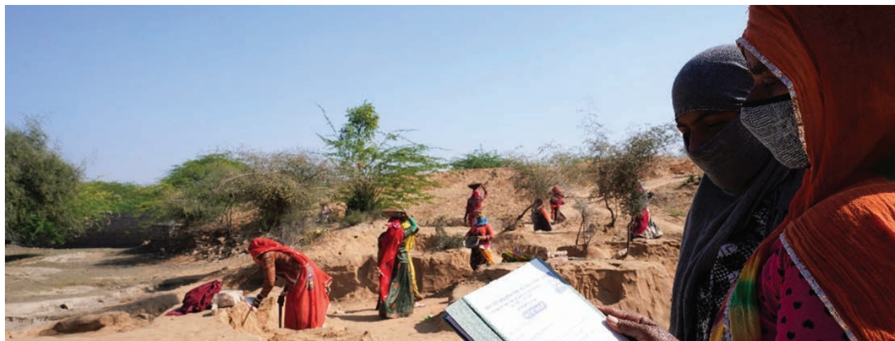
MGNREGA workers are monitoring the work progress during a farm pond construction project under WASCA in village Khaliya, Rajasthan (© Travelling Tripod Films)
